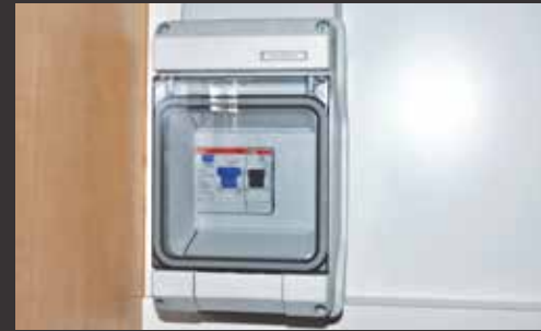
Distribution box with RCD and fuse (16 A)
